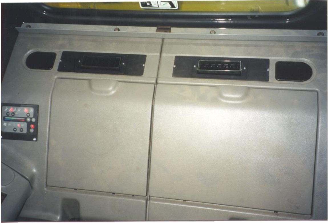
Louvers and controls in place.
